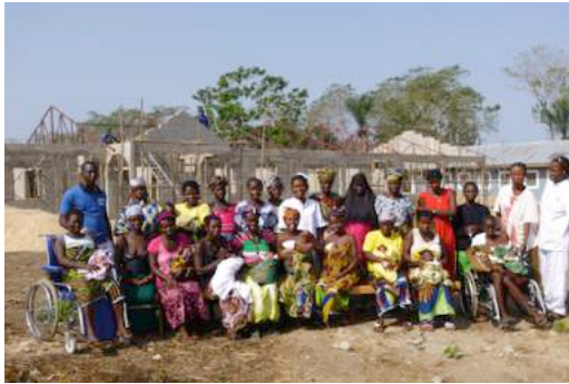
Photo: The maternity ward of the LHMC in construction, with in front Yele mothers and nursing staff.
